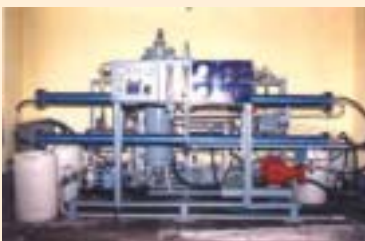
Reverse Osmosis Plant (Capacity : 30 cubic metre per day) set up at Sheelgan village, district Barmer, Rajasthan
